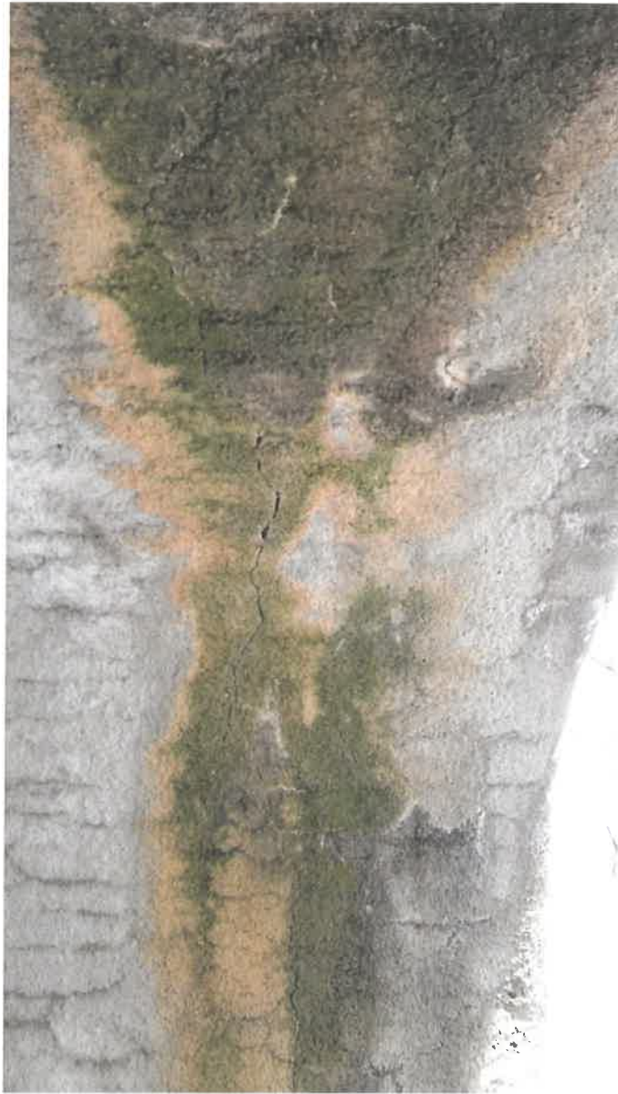
Photo # 6 - Cracking of shotcrete beneath arch of span 2 from north
