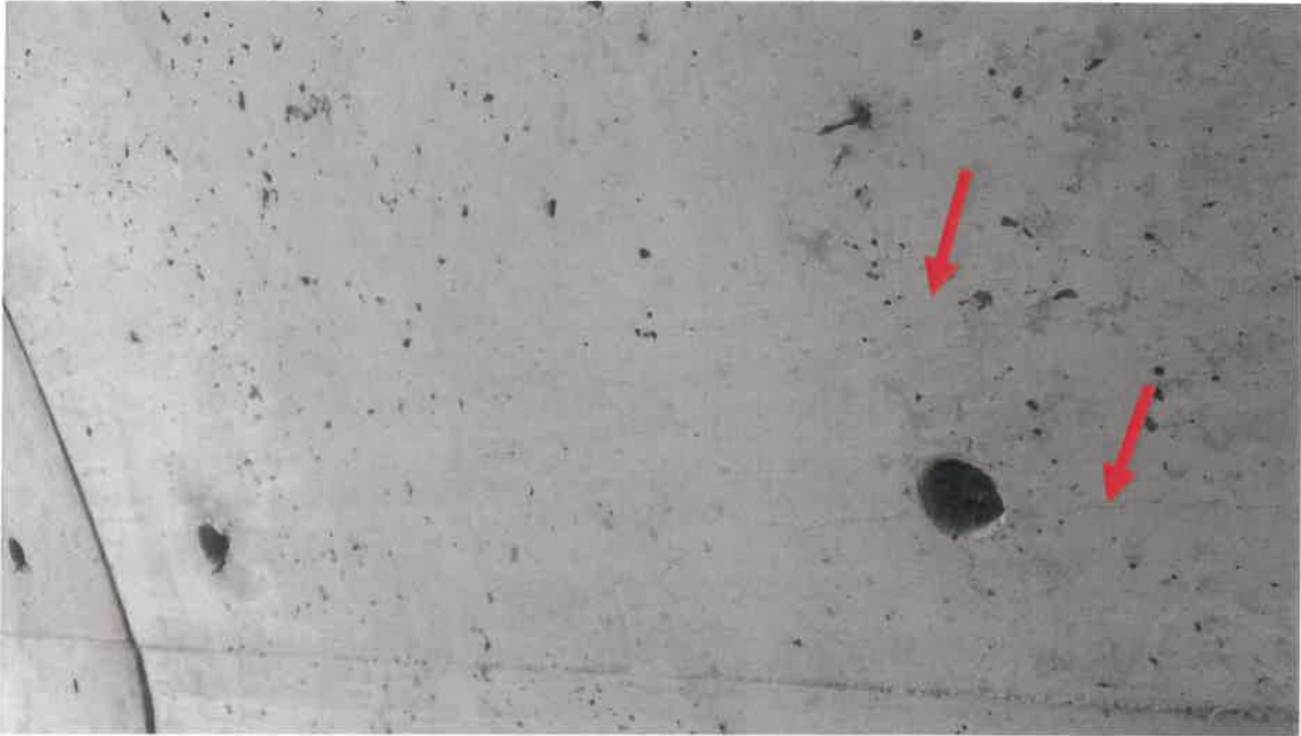
Photo # 5 - Hairline cracks at east end of 2nd arch from upstream end
