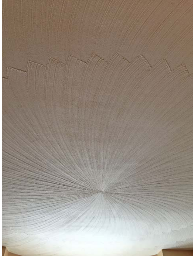
The plaster ceiling in the formal dining room has an ornate swirl pattern.
