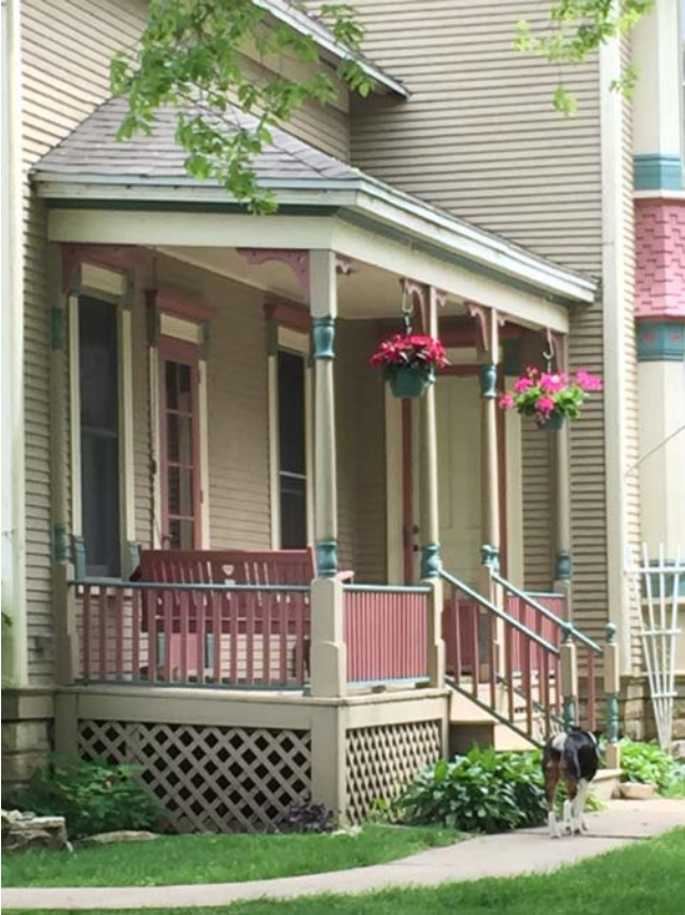
Detail of the porch on the west façade. Note the spindlework porch supports with brackets.
